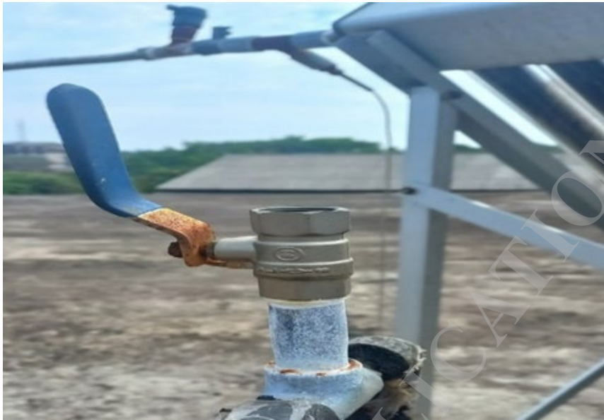
Figure 7. Installed pressure relief valve.
