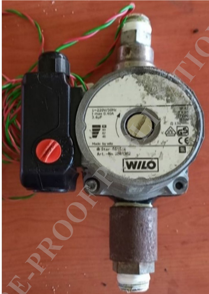
Figure 9. Variable flow hot water pump.
