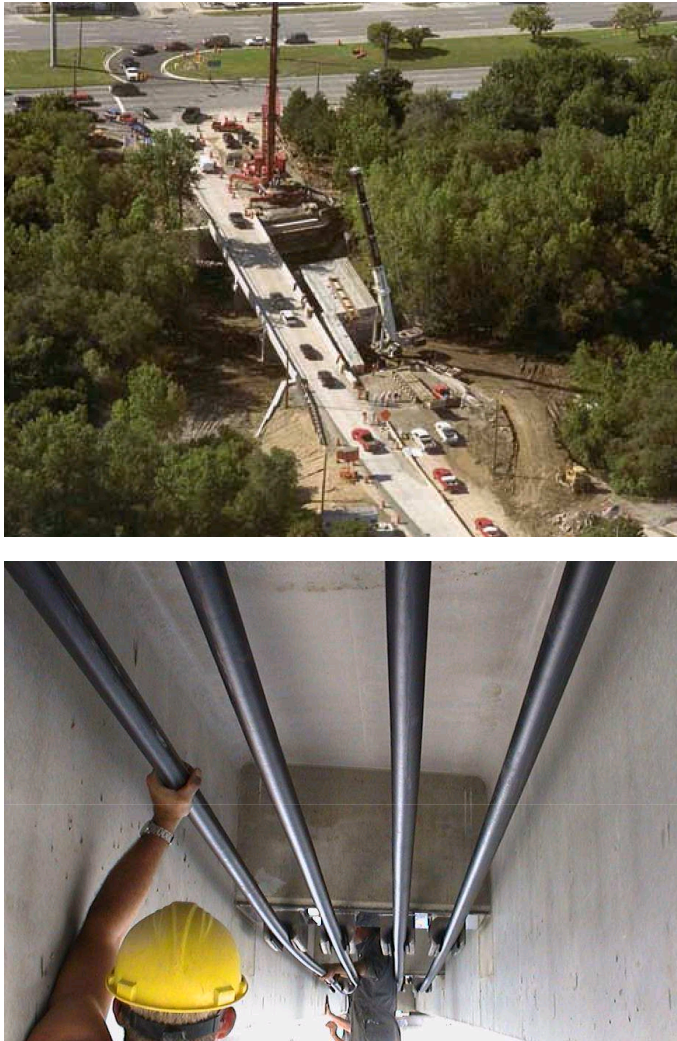
FIG. 2. Execution of the Bridge Street Bridge (top) and fastening of composite tendons (bottom) [4].
